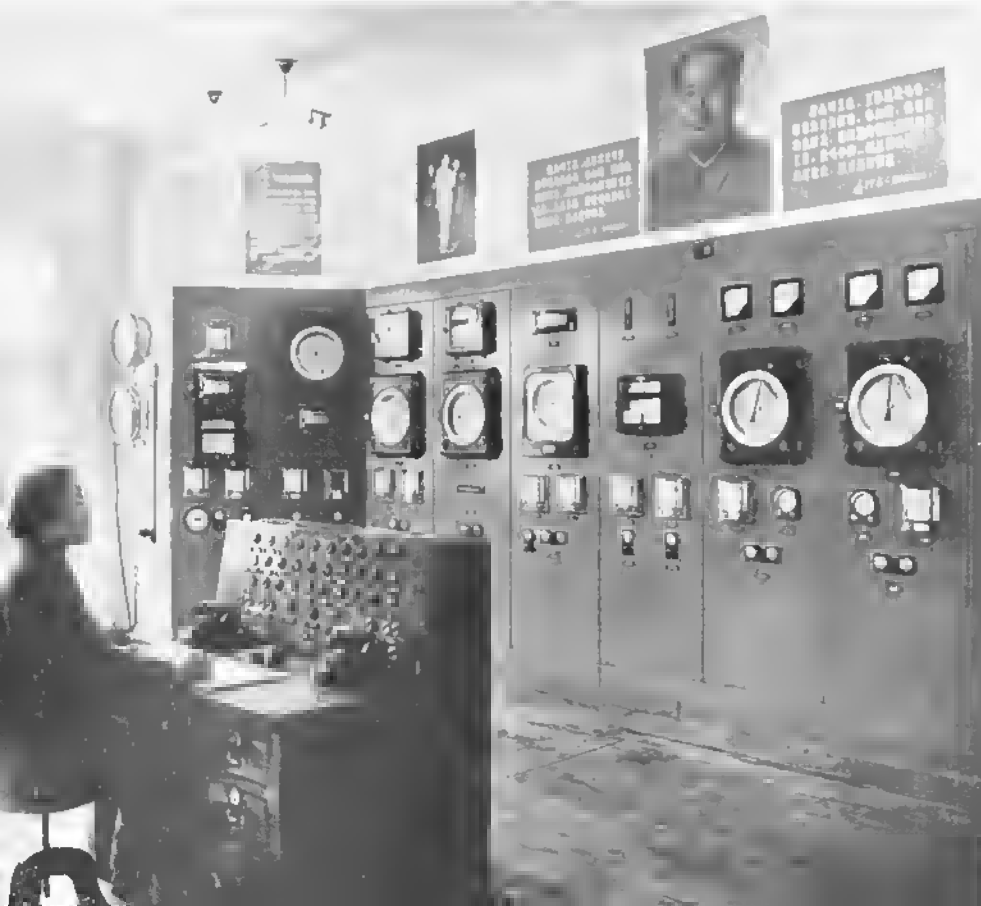
Automatic control board of the urea section.
